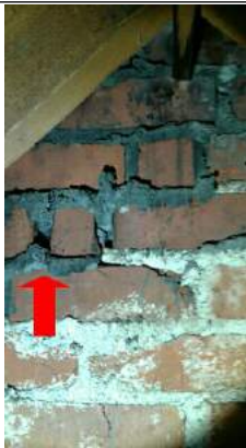
Example of loose mortar joints
