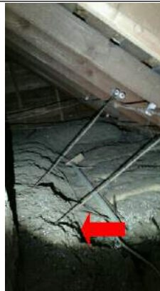
Example of knob and tube in insulation
