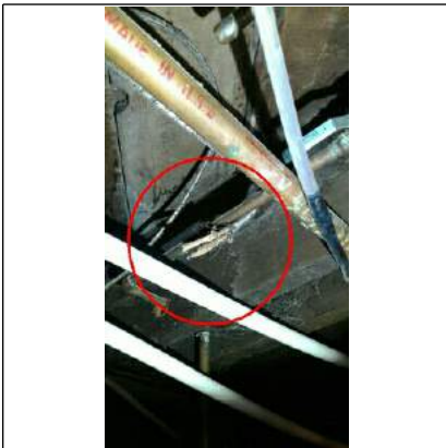
Example of exposed wires
