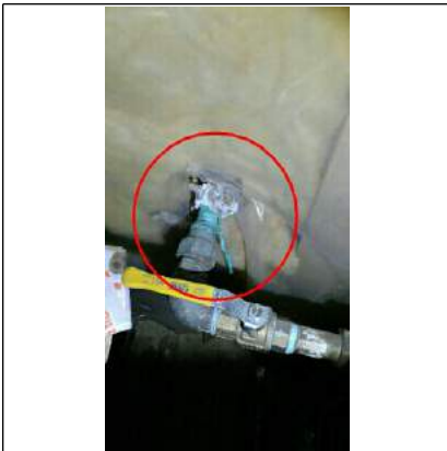
Example of corrosion
