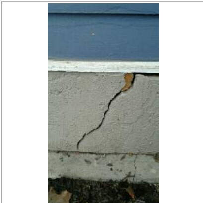
Example of foundation crack
