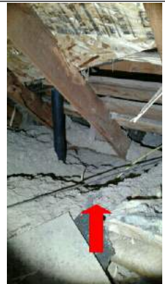
Example of displaced insulation
