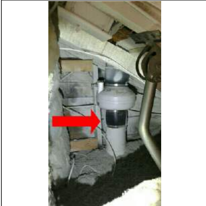
Example of radon mitigation system
